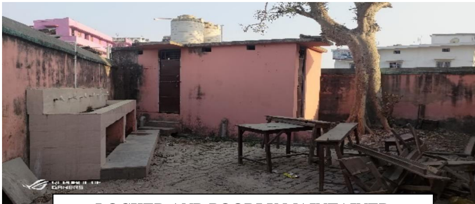
LOCKED AND POORLY MAINTAINED TOILETS AT AMV
