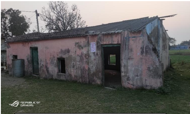
DILAPIDATED BUILDING FOR COOKING MID-DAY MEAL
